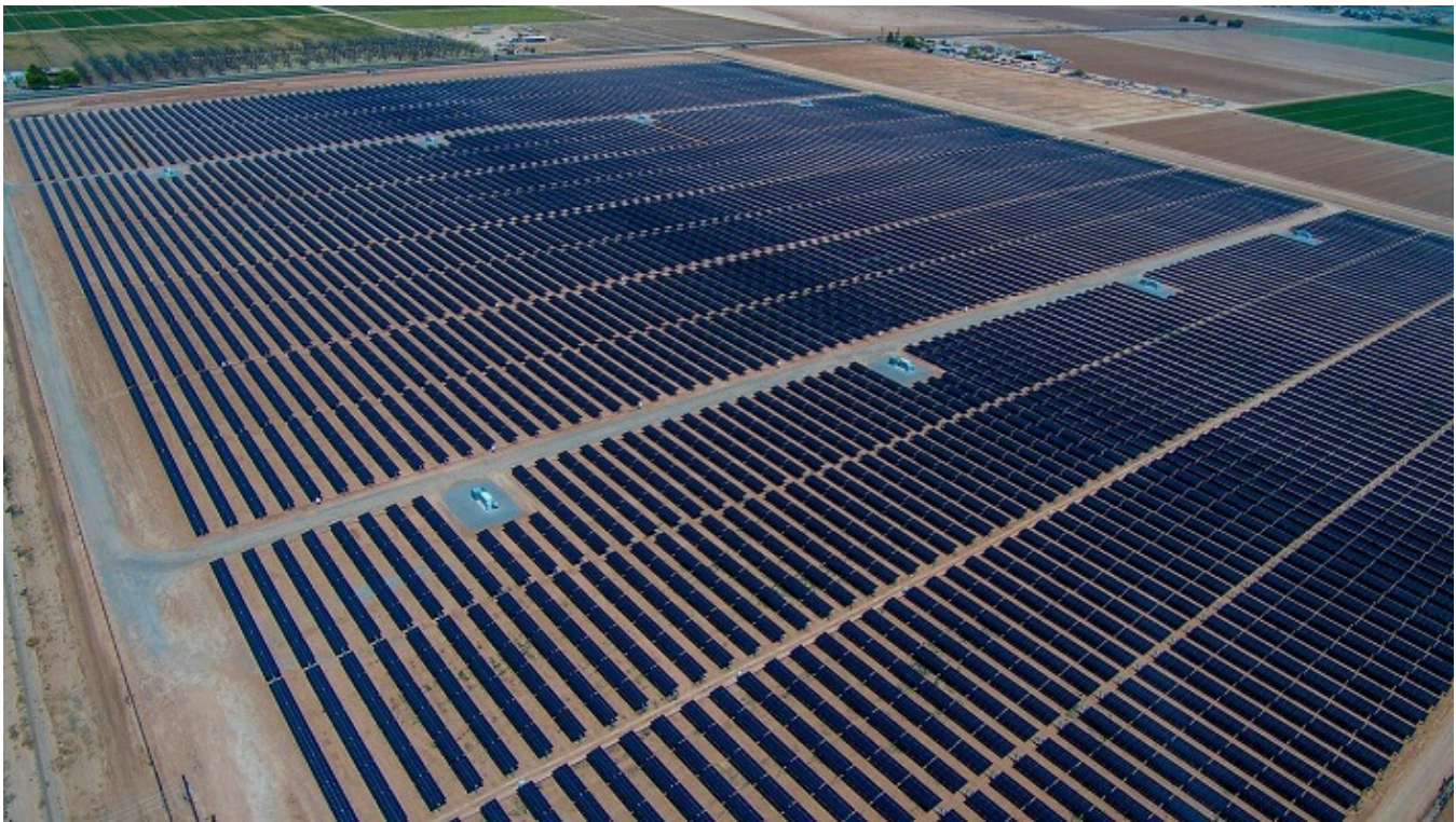
Fig. 1 Utility-scale PV farm (Photo of Pinal Central Solar Energy Center in Arizona).
