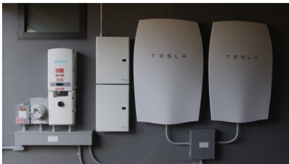
Fig. 3 Residential energy storage (Image: Tesla)
